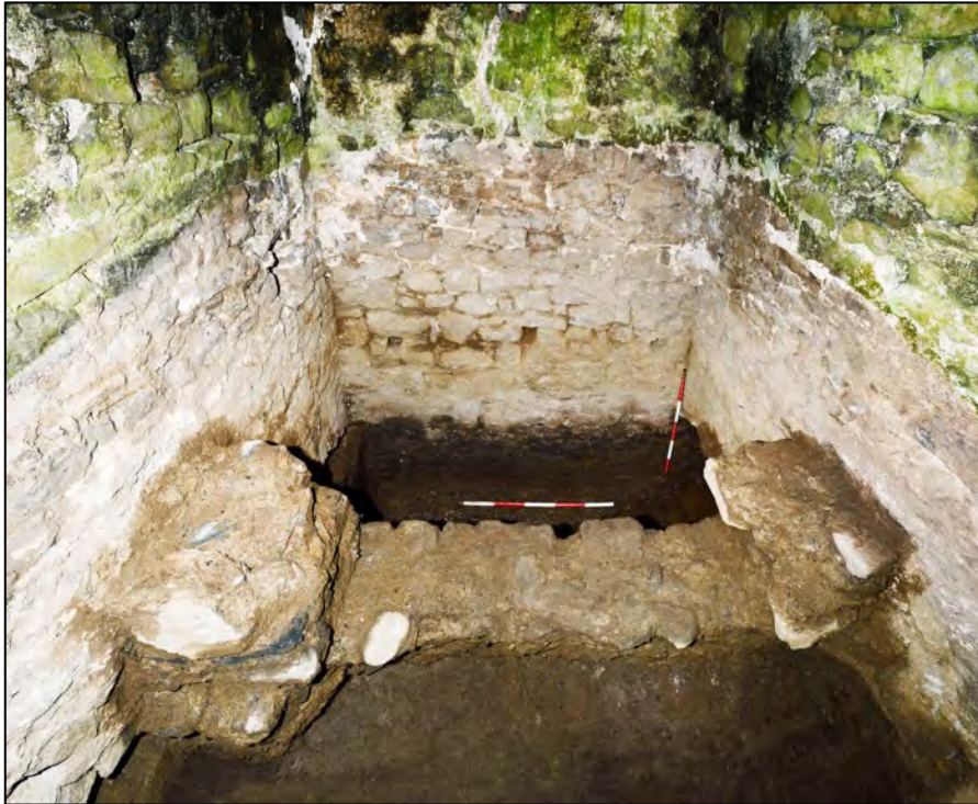
Figure 28: Latrine structure in the interior of the service tower (photo: John Sunderland).
